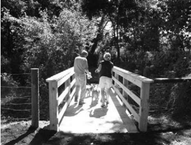
Eagle Scout candidate Jake Yates from Scout Troop 962 constructed an 18-foot-long footbridge that serves as the new entrance to the Phillips Farm interpretive trail. Visitors no longer have to negotiate the steep slope at the trail entrance, and erosion from foot traffic is eliminated. Here, hikers and companions enter the farm. We thank Jake for this generous gift to the community.
